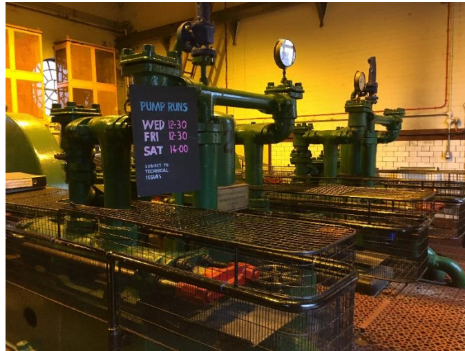
Fig.1 The Pump House
